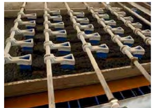
Waste Water Sludge De-Watering
